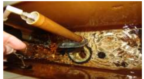
Worn toilet parts
