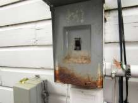
Rusted dead front and missing screw at main panel
