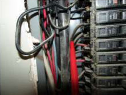
Two knob and tube wires on breakers in house
