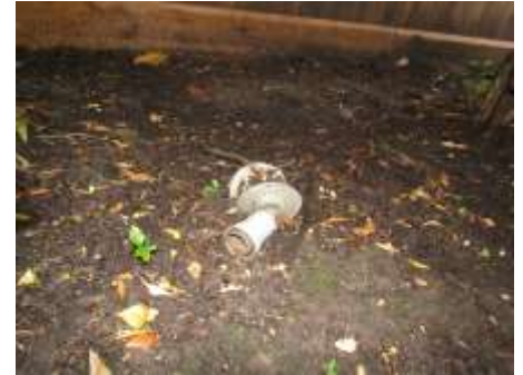
Broken landscape lights
