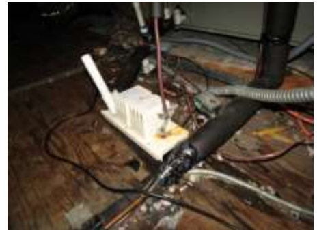
Water leak off first level HVAC drain pump
