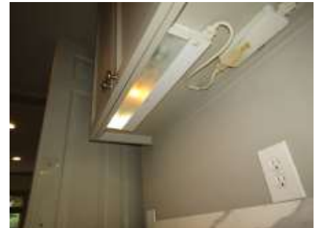
Several under cabinet lights burnt out
