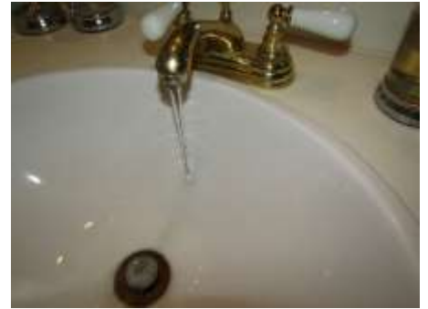
Weak pressure at lavatory
