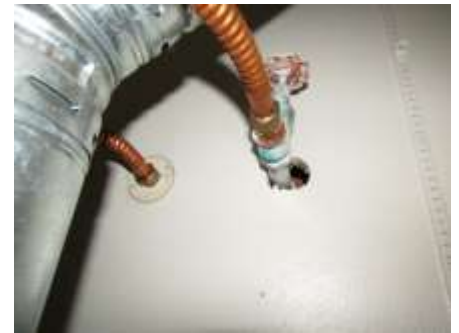
Corrosion on quarters water heater stop and fittings
