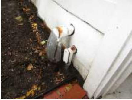
Rusted LB and conduit at garage to house
