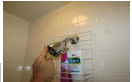
Loose third level shower arm
