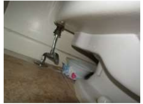
Water leakage under toilet
