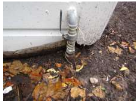
Rusted gas from garage to house
