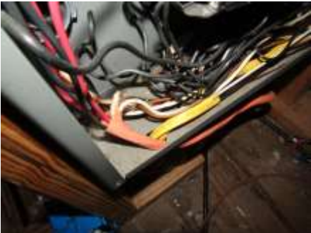
Missing connector of cable wire on panel in attic
