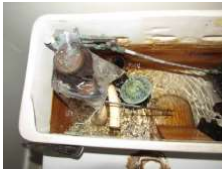
Worn parts for toilet
