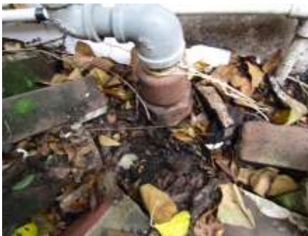
Rusted gas pipe at grade
