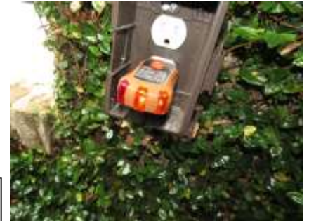
Not GFCI at exterior outlets
