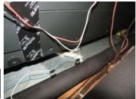
Water in second/third level HVAC pan
