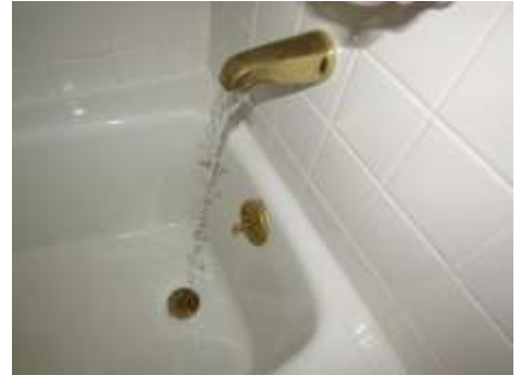
Weak hot water in tub
