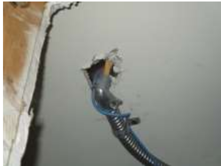
Missing junction box for male electrical in upper elevator
