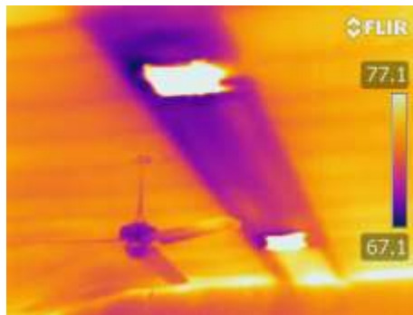
Heat images from heater mode in operation
