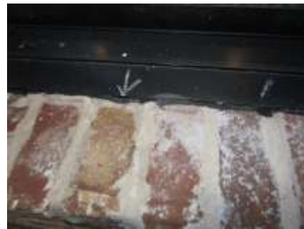
VOIDS in exterior window and sill caulk
