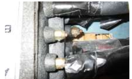
Missing insulation on second level manifold
