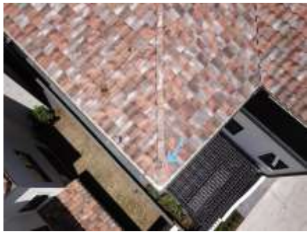
Broken tile at southwest hip
