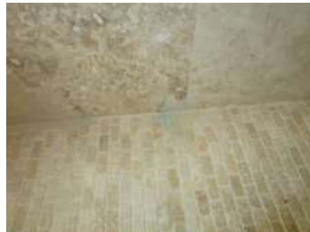
Stained tile in master shower
