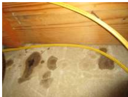
Water on ceiling of third level HVAC from condensation leak
