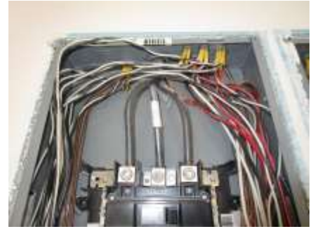
Strap loose wires on panel
