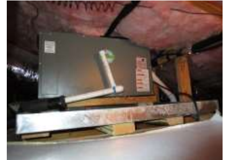
Incomplete insulation on dehumidified unit drain in attic
