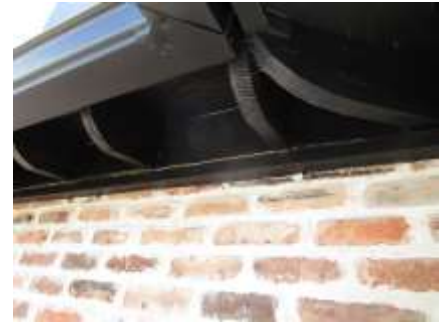
Loose trim at upper southwest area
