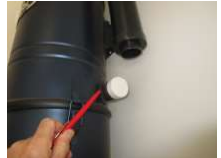
No external exhaust and missing connection off unit
