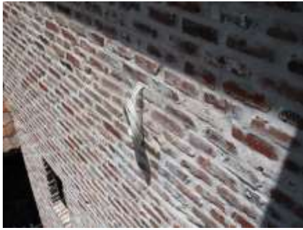
Exposed cable at upper southwest wall
