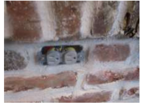
Missing cover on patio outlet
