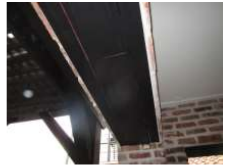
Uneven wood at rear patio
