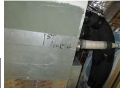
No emergency pans under all five HVAC units
