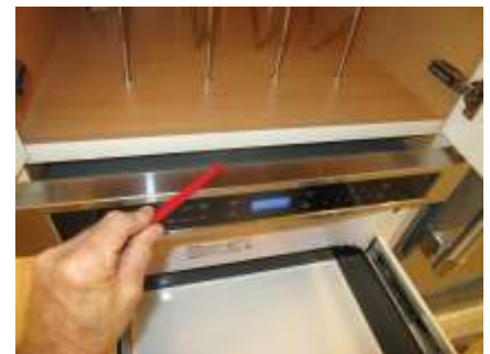
Loose microwave in cabinet
