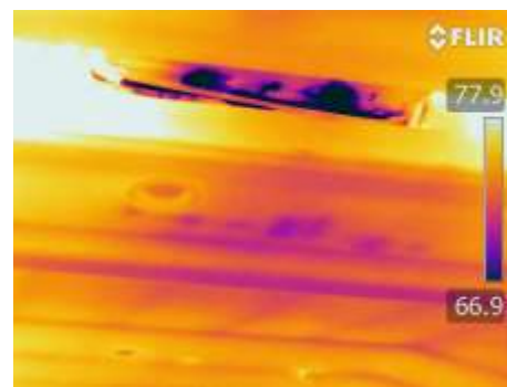
Water leakages on ceiling and 3rd level HVAC equipment
