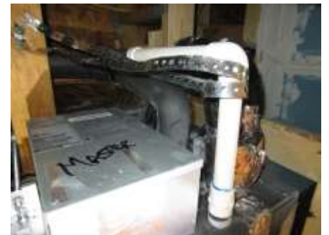
Vibration off master HVAC air handler
