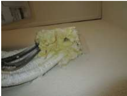
Poor foam installation at HVAC utilities
