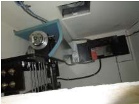
No air register in elevator chase
