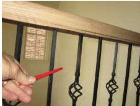
Loose iron balusters in stairs
