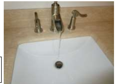
Weak hot water at powder bathroom lavatory
