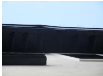
Damaged east gutter
