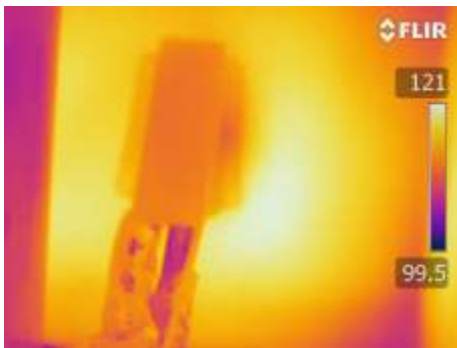
121 degrees at east side enclosure for A/C split systems
