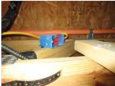
Open junction box in laundry room ceiling
