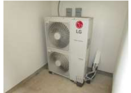
HVAC units installed in area with limited air
