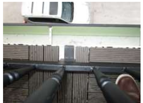
Missing tile paver at third level balcony
