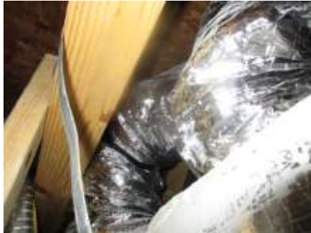
1" clearance not at ducts
