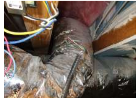
Exposed cable wires off first level south HVAC
