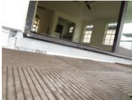
Missing vertical support under third level balcony threshold
