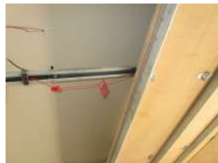
Garage door operator not connected
