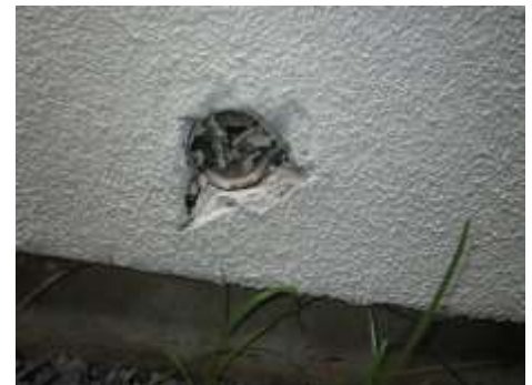
Missing ell for laundry room drain
