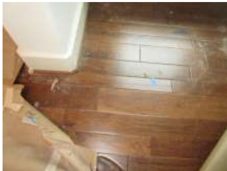
Uplifted wood flooring in third level
