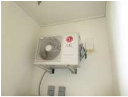
Vibration in wall from mounted HVAC
