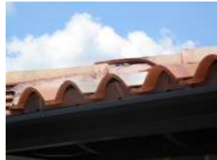
Broken upper southwest tile
