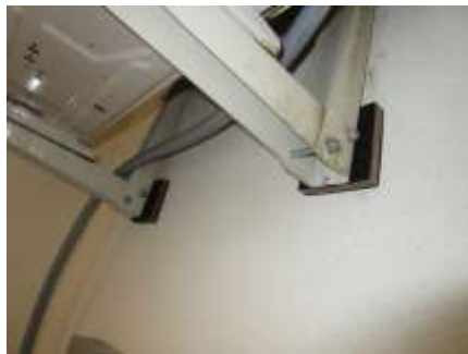
Poor installation of HVAC unit on stucco wall
