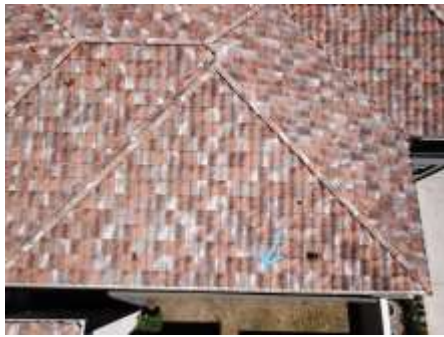
Hairline cracks at southwest tiles
