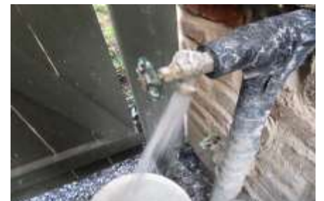
Missing backflow devices
