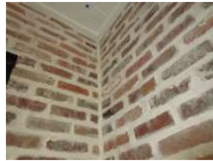
Vertical corner wall cracks on patio
