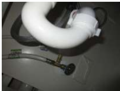
Third level dishwasher and ice maker on hot piping and no separate stops
