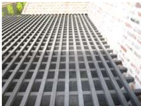
Worn stain on top of patio arbor
