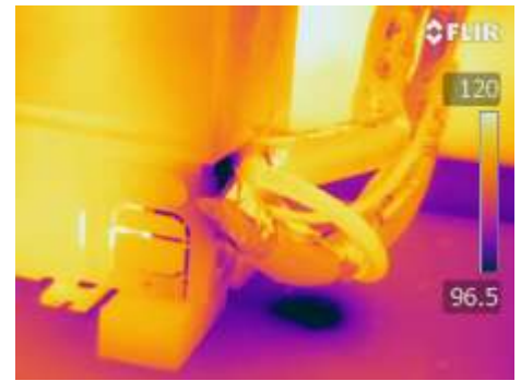
Water off HVAC exterior split system on east side
