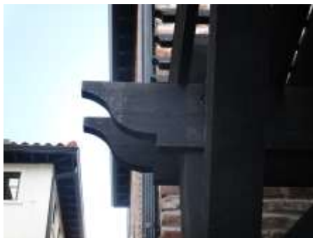
No protection on top of wood
