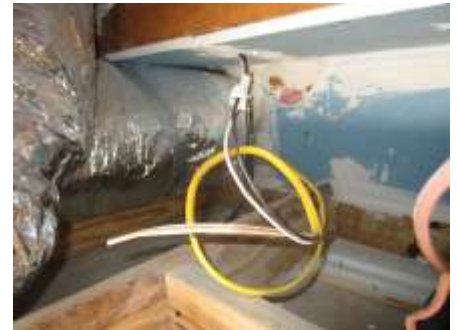
Exposed wires off first level south HVAC
