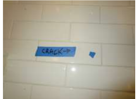
Cracked tile in laundry room
