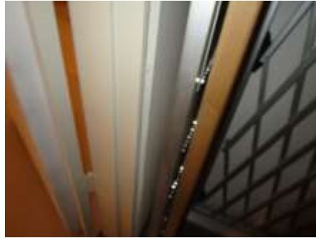
Incomplete trim for wall inside elevator
