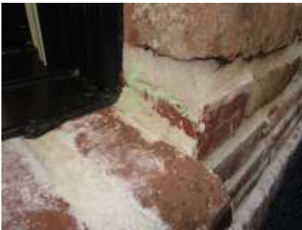
VOIDS at brick and windows
