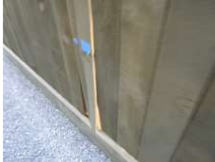
Loose east side fence pickets
