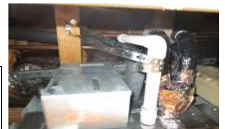
Odd emergency drain installation off HVAC units in ceilings
