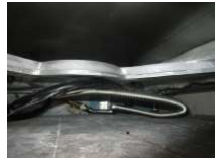
Limited access to range gas stop valve
