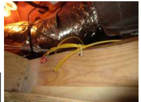
Exposed, loose and unused wires in third level attic
