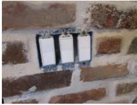
Missing rain and damp proof cover on patio switches
