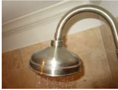
Showerhead leak on second level shower
