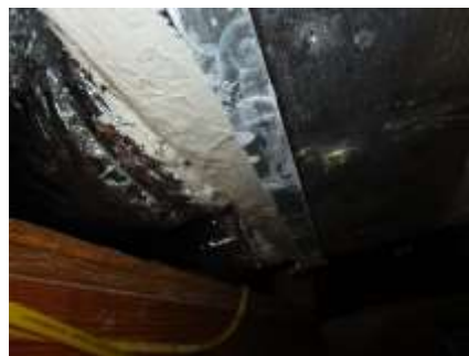
Excess condensation drips off third level HVAC
