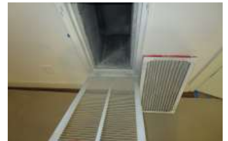
Possible undersized return air for master HVAC
