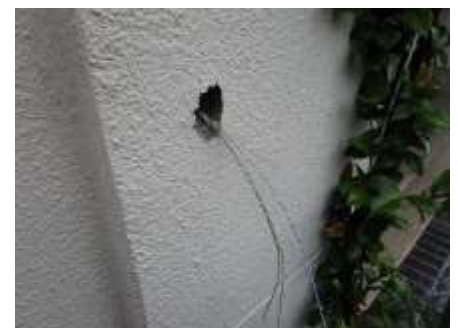
Missing rear south doorbell
