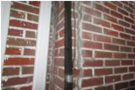
Previous repairs to brick and separation
