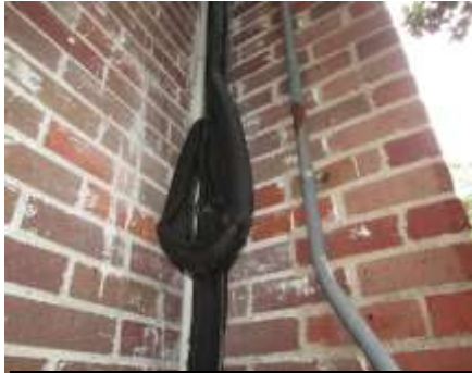
Exposed refrigerant line and torn insulation
