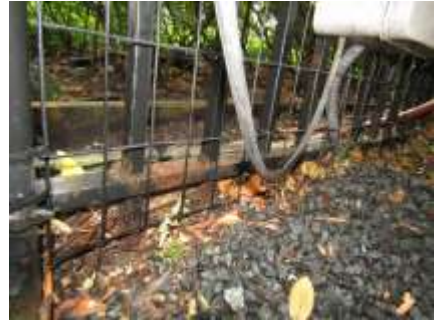
Rusted lower fence and gate
