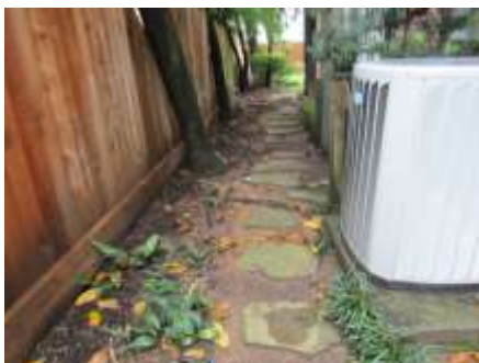
No area drains at east side
