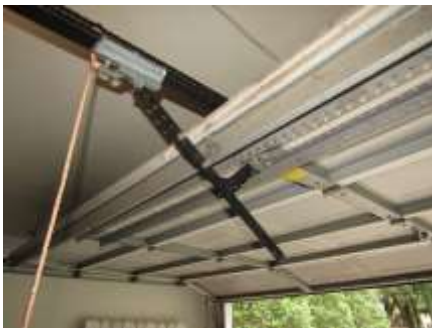
Damaged top of garage overhead door panel
