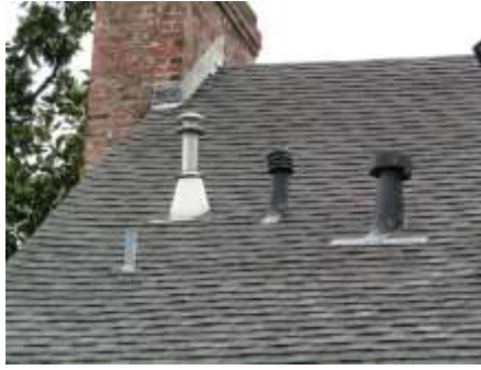
Gas vent pipe projections for previous or existing water heater(s)
