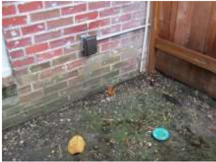
Stains and vegetation
