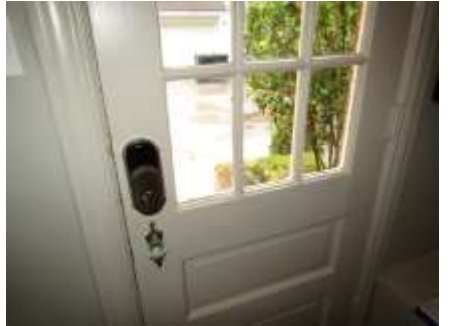
Glazing not tempered at doors
