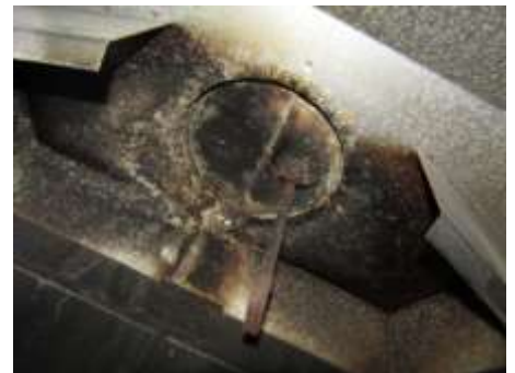
Rust and creosote at master fireplace
