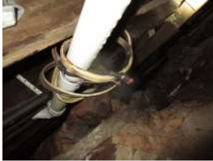
Exposed and energized electric cables
