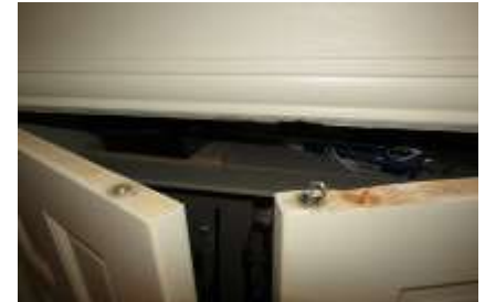
Broken double door roller balls
