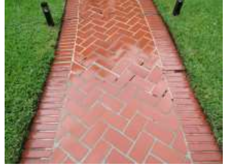
Broken front walkway pavers
