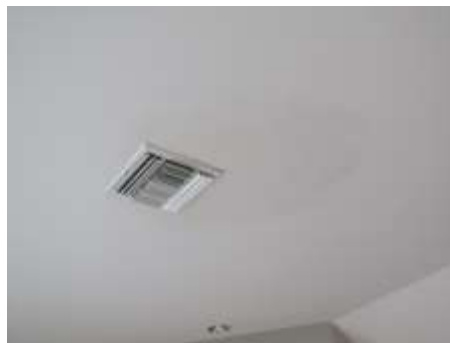
Wet master bedroom ceiling
