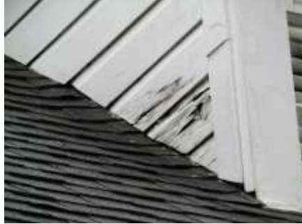
Damaged wood off front dormers
