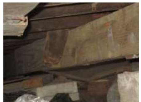
Loose support under beam
