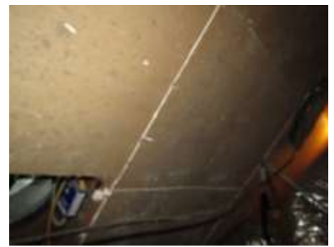
Black organic substance in third level attic
