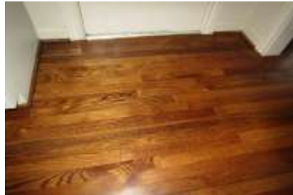
Cupped hardwoods at west door
