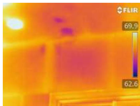
Water images on ceiling and wall of 2 nd level north bathroom
