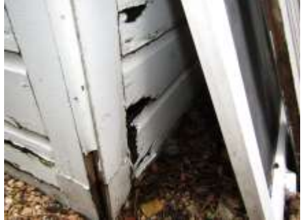
Damaged wood at garage
