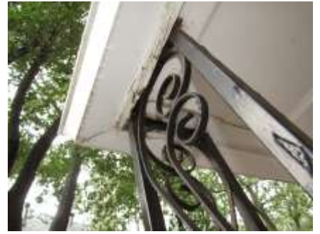
Rotted and damaged wood off west roof cover
