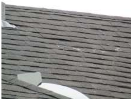
Worn granules at upper rear shingles
