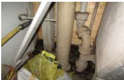
Daylight, water and damages in garage
