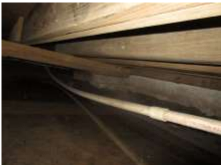
Loose PVC piping under east house
