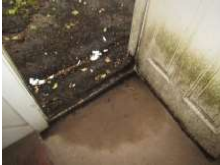
High soils and damages at side quarters door
