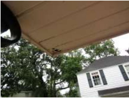
Rotted wood off rear south roof cover
