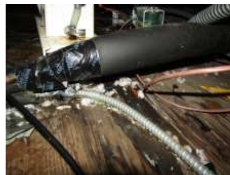
Water on attic deck from first level HVAC drain pump
