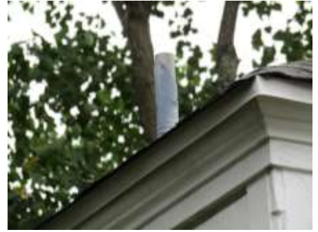
Damaged lead roof jack
