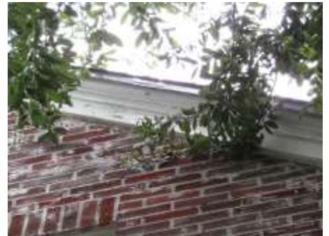
Tree branches and damaged shingles
