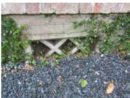
Low west vent and ivy over screen
