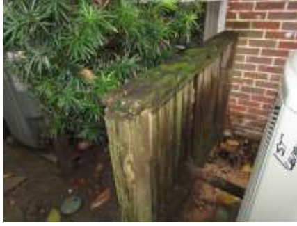
Damaged east side fence
