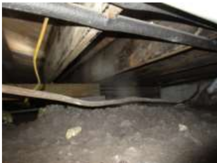
Loose electric wires under house
