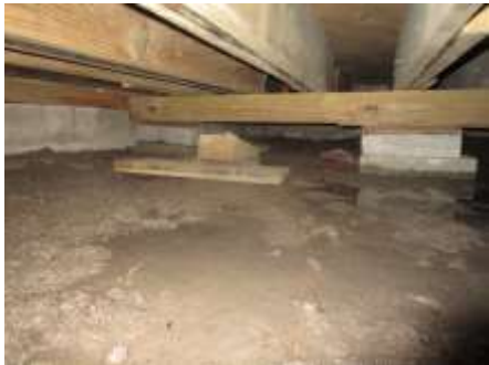
Wood debris under east house
