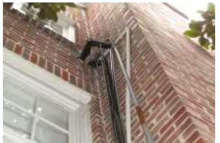
Loose, exposed and rusted piping
