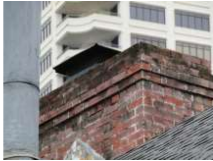
Stained brick off chimney
