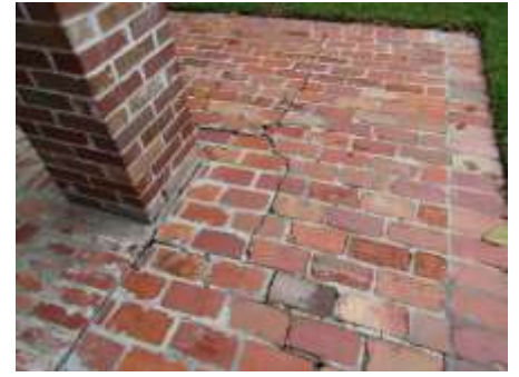
Broken rear east pavers
