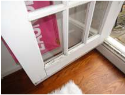
Damaged upper balcony door and casing
