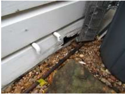
Damaged wood at garage
