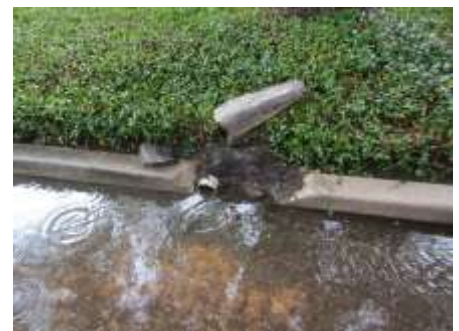
Clogged drain at curb and broken curb
