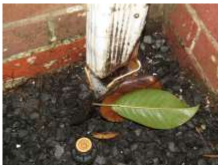
Clogged rear east gutter drain
