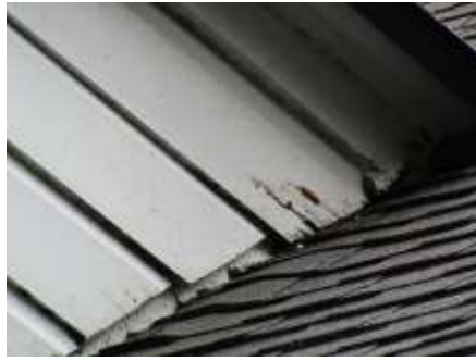
Rotted wood at front upper dormers
