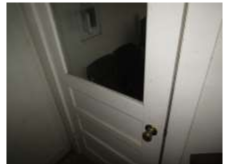
Glazing not tempered at garage quarters
