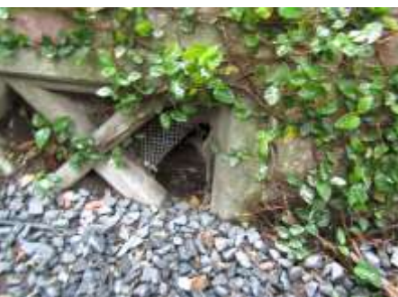
Torn west vent screen
