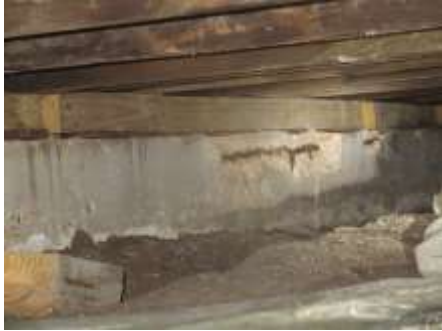
Exposed rebar inside west concrete stem wall
