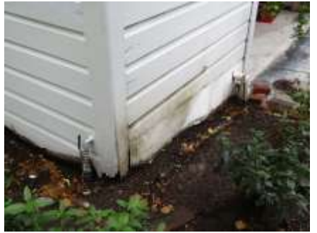
Damaged siding and trim and metal flashing at front garage
