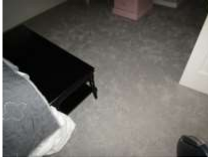
Squeaking sub flooring
