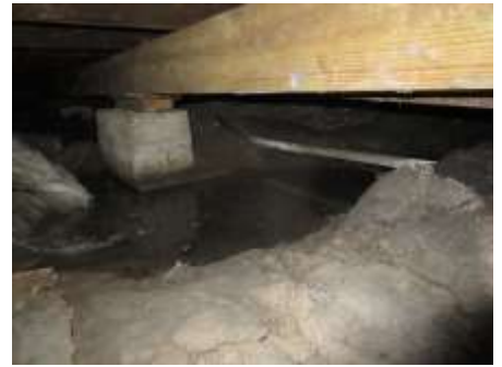
Water under center crawl space
