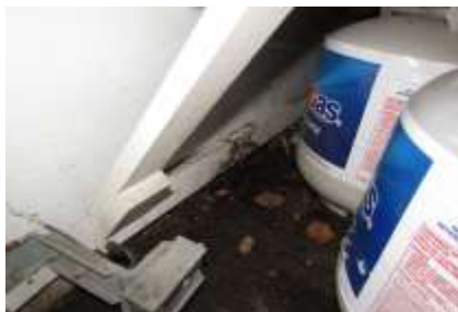
Water inside garage
