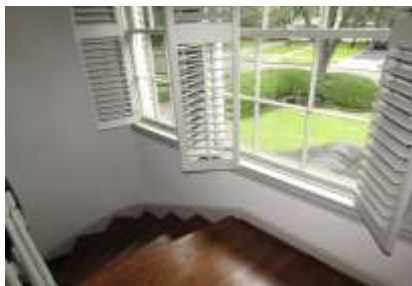
Glazing not tempered at stairs
