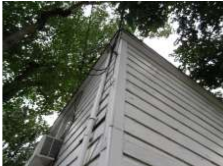
Tree branches on quarters roof
