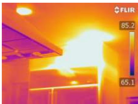
Typical image of heat off refrigerator unit in kitchen
