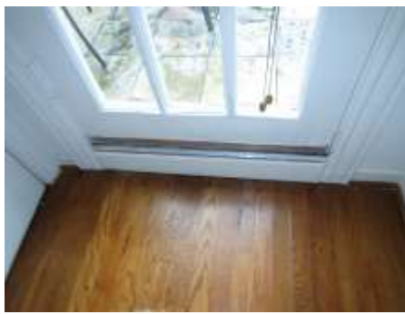
Stains inside upper rear west balcony door
